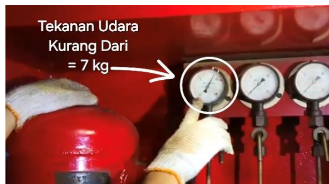
Gambar 6. Manometer di panel box air receiver Sumber: Dokumen pribadi
